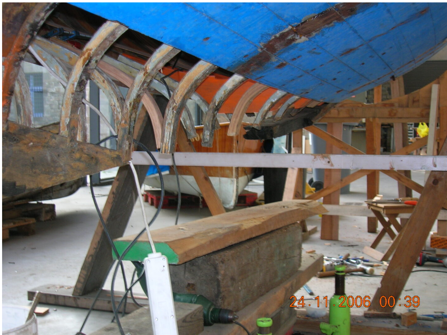
The restoration of the Drac required the keel to be completely rebuilt. Photo: MMB.
